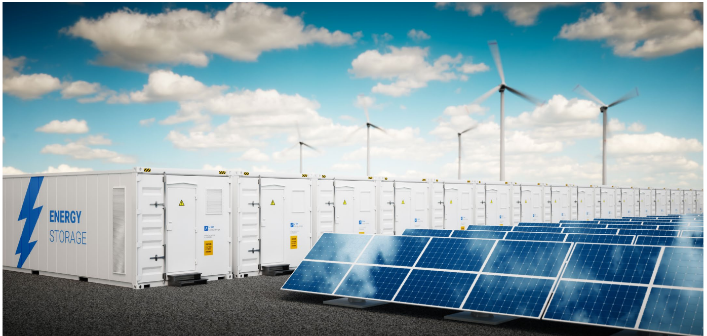
Renewable energy power plants - photovoltaics, wind turbine farm and battery container.
