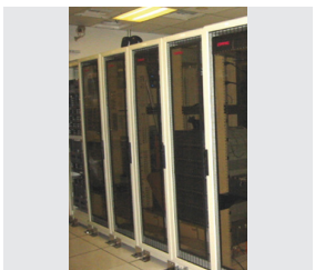
Am Boden verankerte Server Racks
