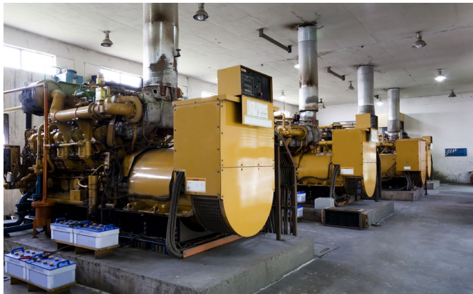
Diesel Engine Driven Emergency Generators
